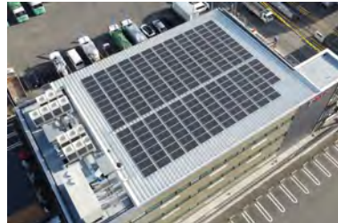
Solar power generation panels installed on the roof
